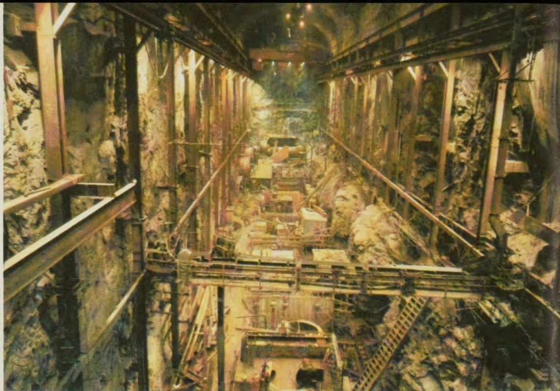
Underground Power House at Manapouri hewn out of solid rock 700 ft. below a control building on the shore of Lake Manapouri. The underground power house, shown here under construction, houses 7 turbines each driving a 100,000 kw generator. Power generated will be supplied to the Comalco aluminium smelter at Bluff.
